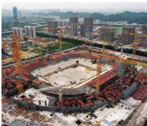
The construction site of Guangzhou Evergrande Soccer Stadium in September 2021. Developed by China Evergrande Group
