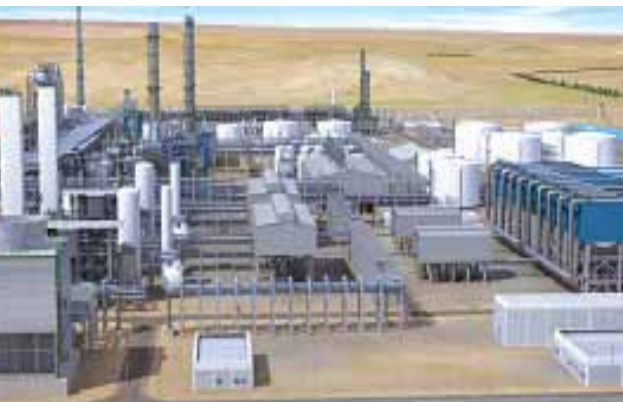
Construction of the Oltin Yo'l GTL plant near the Shurtan Gas Chemical Complex
