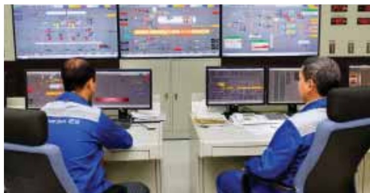
Talimarjan power plant
