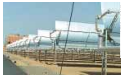
Ouarzazate thermosolar project, Morocco
