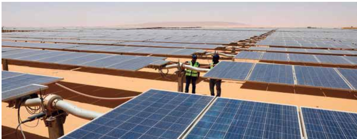
... and fire The Benban Solar Energy Park in Aswan
